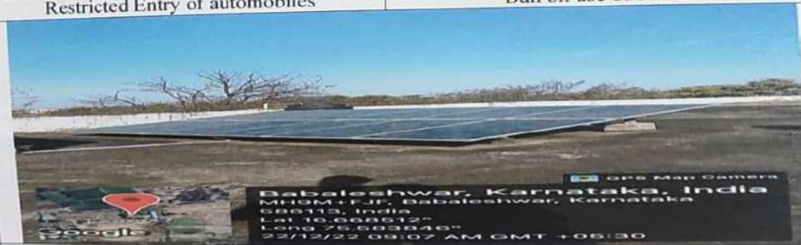
Solar energy panels Installed on rooftop of the college building
